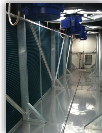
Interior view of the equipment: Great accessibility
