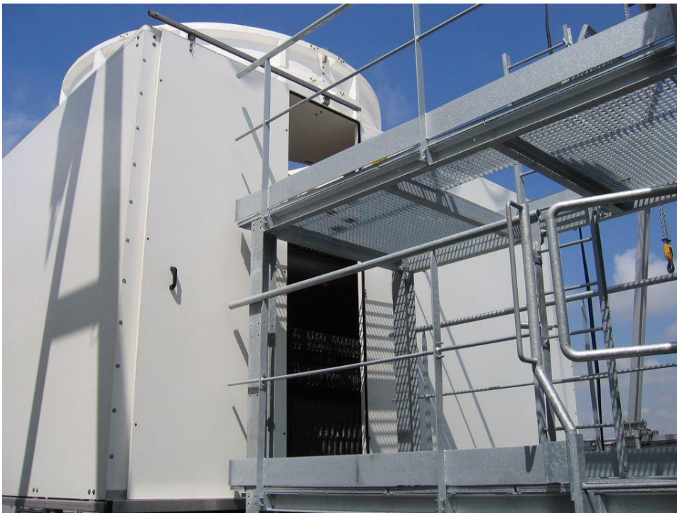
Large sliding door for access to the exchange surface, dispersers, droplet separators and motor-reducer-fan unit.
