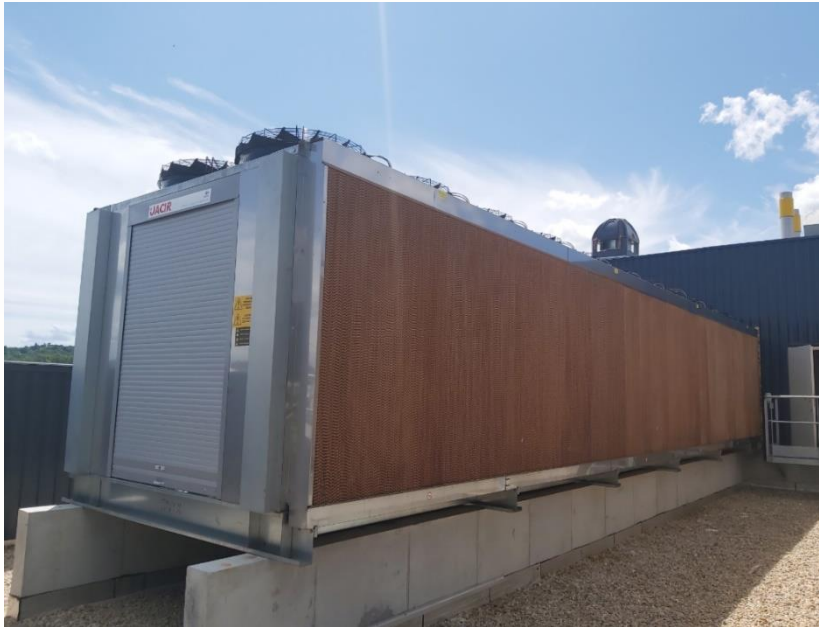
Containment and refrigerant fluid recovery device in case of potential leaks
